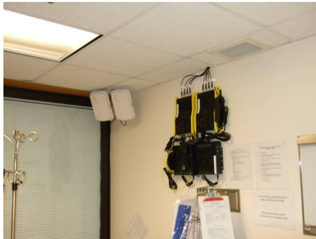
Figure 11: Picture - 3C12 Storage 2
